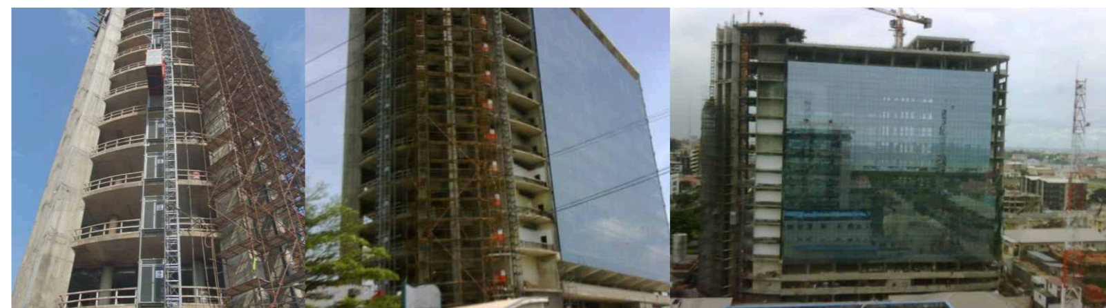
PROPOSED 15 STOREY ULTRA MODERN OFFICE BUILDING , FF MILLENNIUM VICTORIA ISLAND, LAGOS ONGOING PROJECT SINCE 2009
